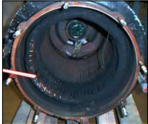
Figure 21. Overall discoloration of the stator winding—usually indicates excessive temperature. Check load, power supply and cooling.
