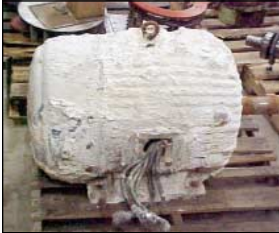
Figure 15. Motor with blocked cooling ribs.
