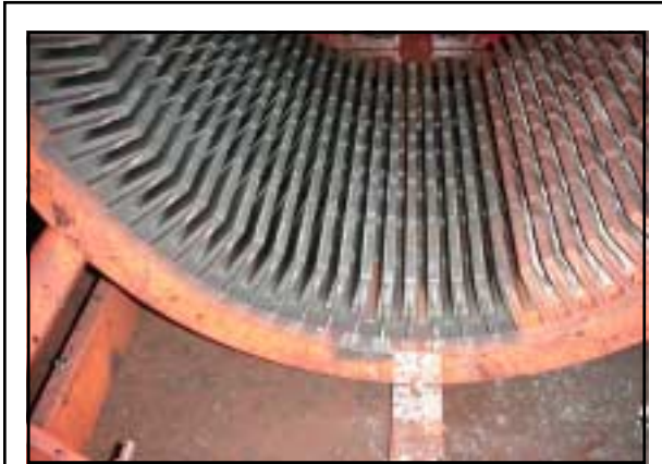
Figure 24. This core has been partially cleaned by using a high-pressure washer to remove the slot insulation debris.
