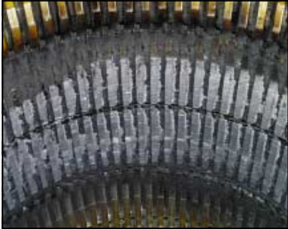
Figure 19. A major core rub; not repairable unless core is dismantled and repaired.
